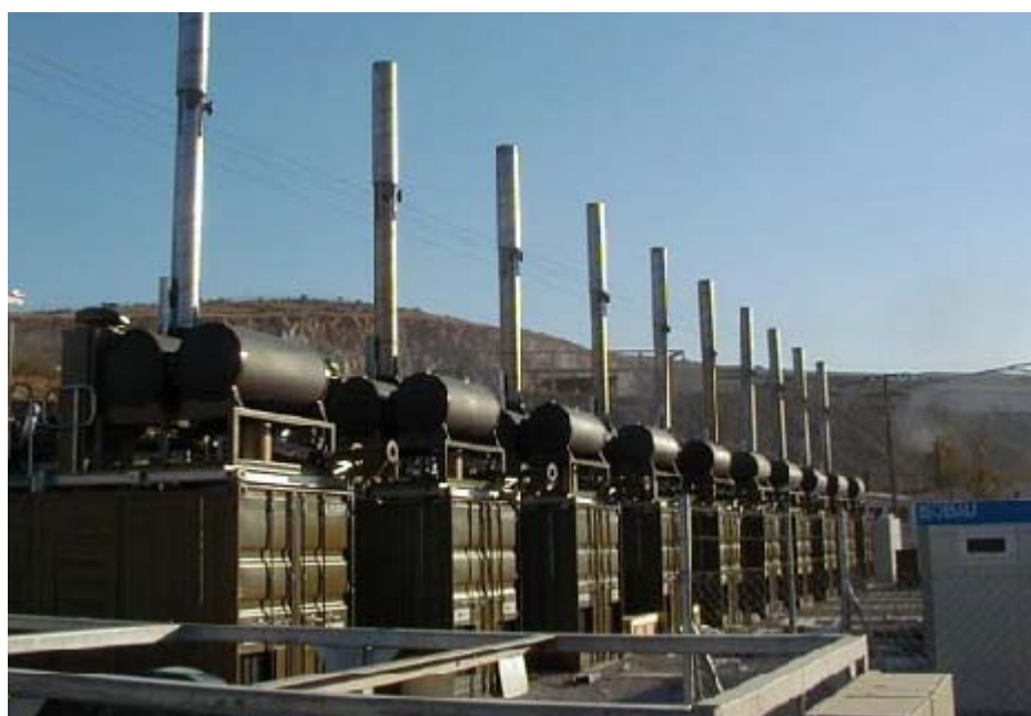
A biogas plant with 10 parallel fermenters
