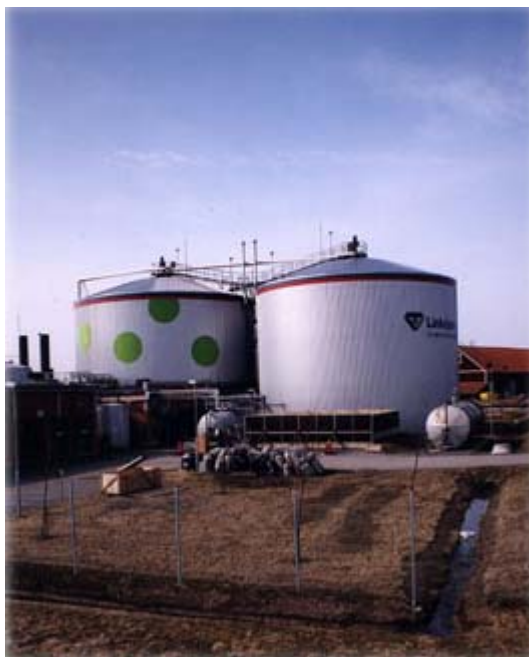
Biogas plant with two anaerobic digesters
